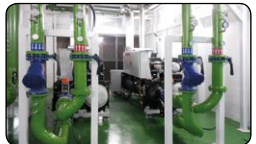
Industrial application, installed in Spain with Turbocor compressors, 840kW
