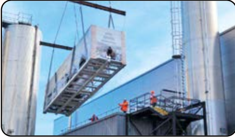
* Chiller installed in UK, 1070 kW
