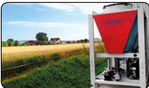
* Modular reversible air to water heat pump installed in Switzerland for space heating/cooling. 105kW @ +45°C LWT
