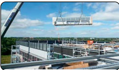
* Chiller installed in Dusseldorf, Germany, 820 kW
