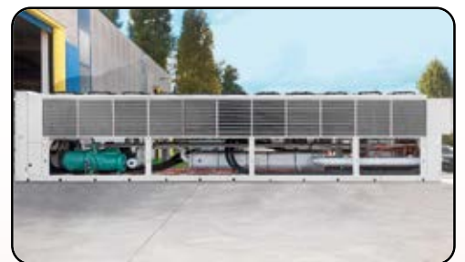
Free-cooling chiller, 1240kW * 460/3/60 UL, ASME evaporator Installed in USA for Data Center
