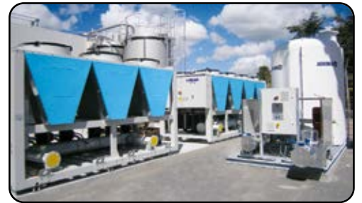
Chillers installed in France, total cooling capacity 1155 kw
